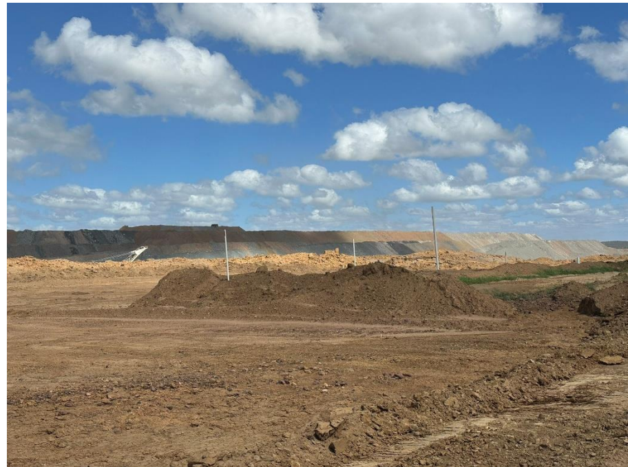
Photo 18: soil stockpile (10 December 2025) (not the best example of how we store topsoil though – this is just a temporary dozer push stockpile that is waiting relocation to final stockpile placement).
